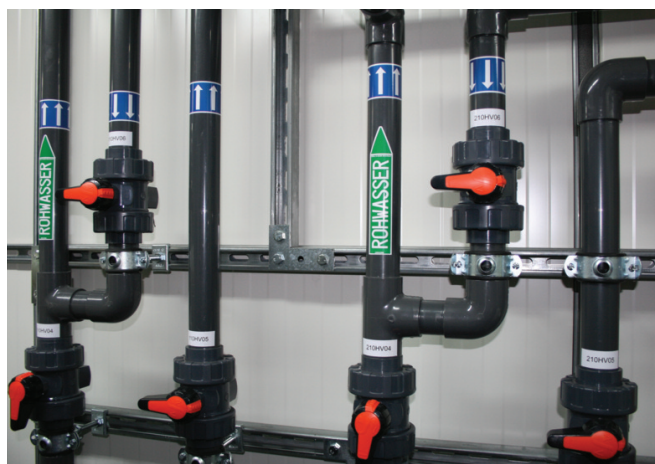
Figure 2: Labels on service water pipes (Source: MULTI-ReUse)
